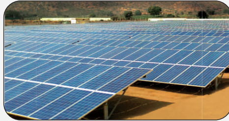
MW EPC SERVICES
