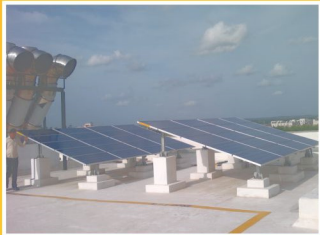
Solar Power Pack
